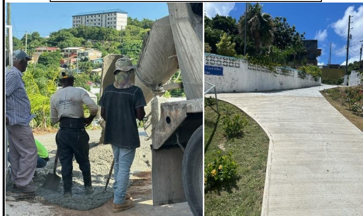
Completion of the walkway from the church to the Cassi Hill Shrine
